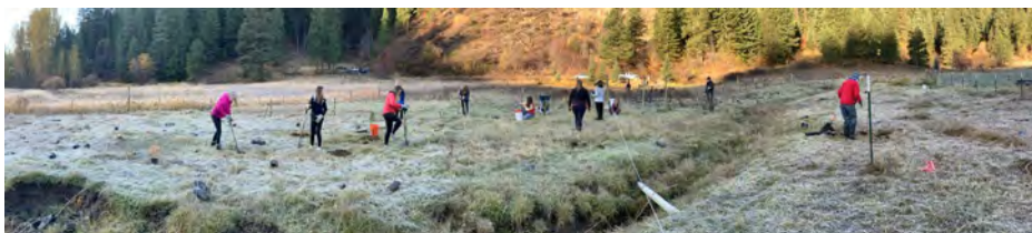
More than 1700 native trees and shrubs were installed in the riparian area along the Little Chumstick this fall to improve water quality and restore wildlife habitat
