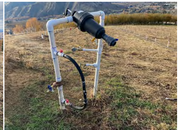
Newly installed water saving pressure reducer and filter for micro and drip irrigation system
