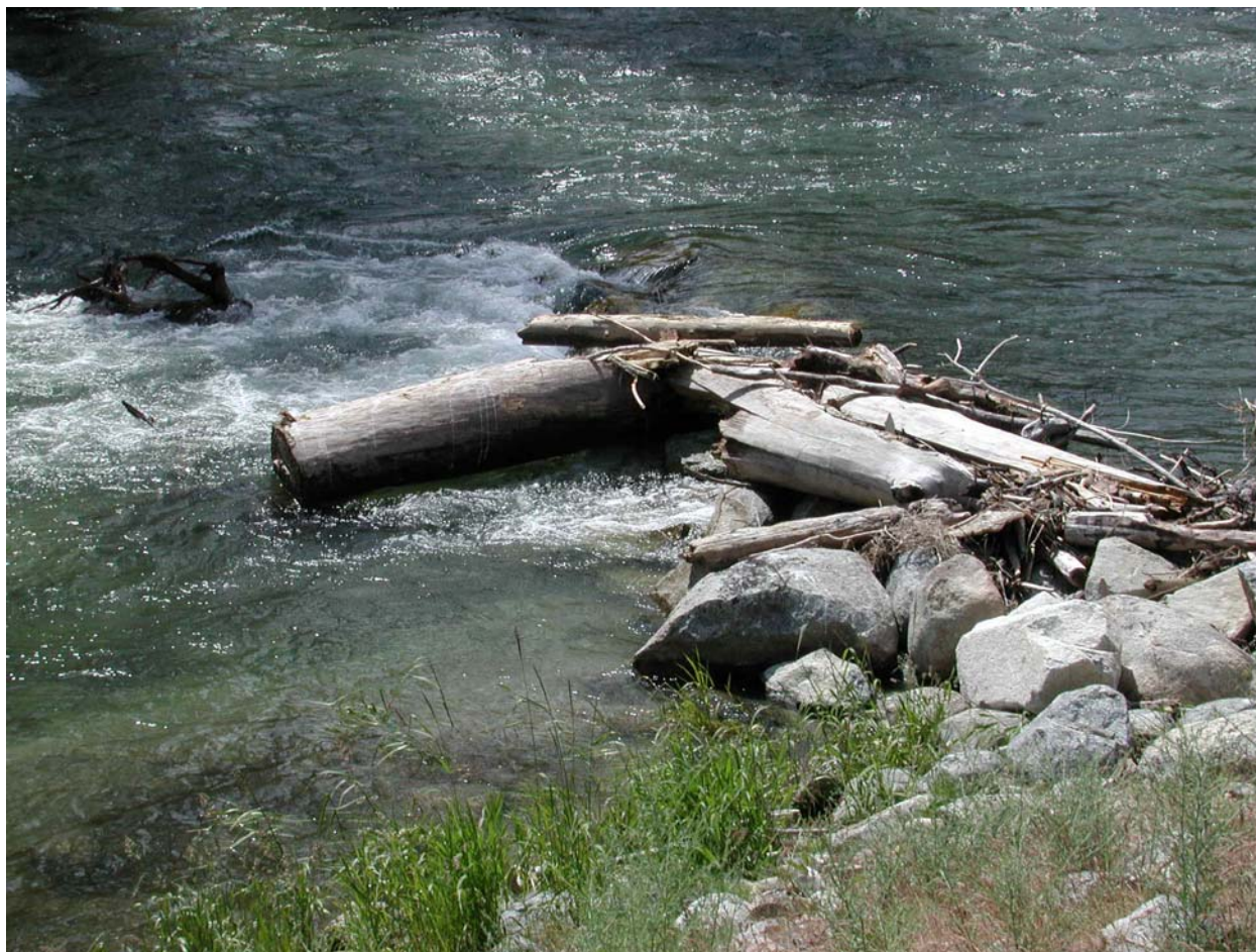
Figure 7-18 One of two large boulder barbs with root wads installed near RM 15 by the BLM during the fall of 2001.
