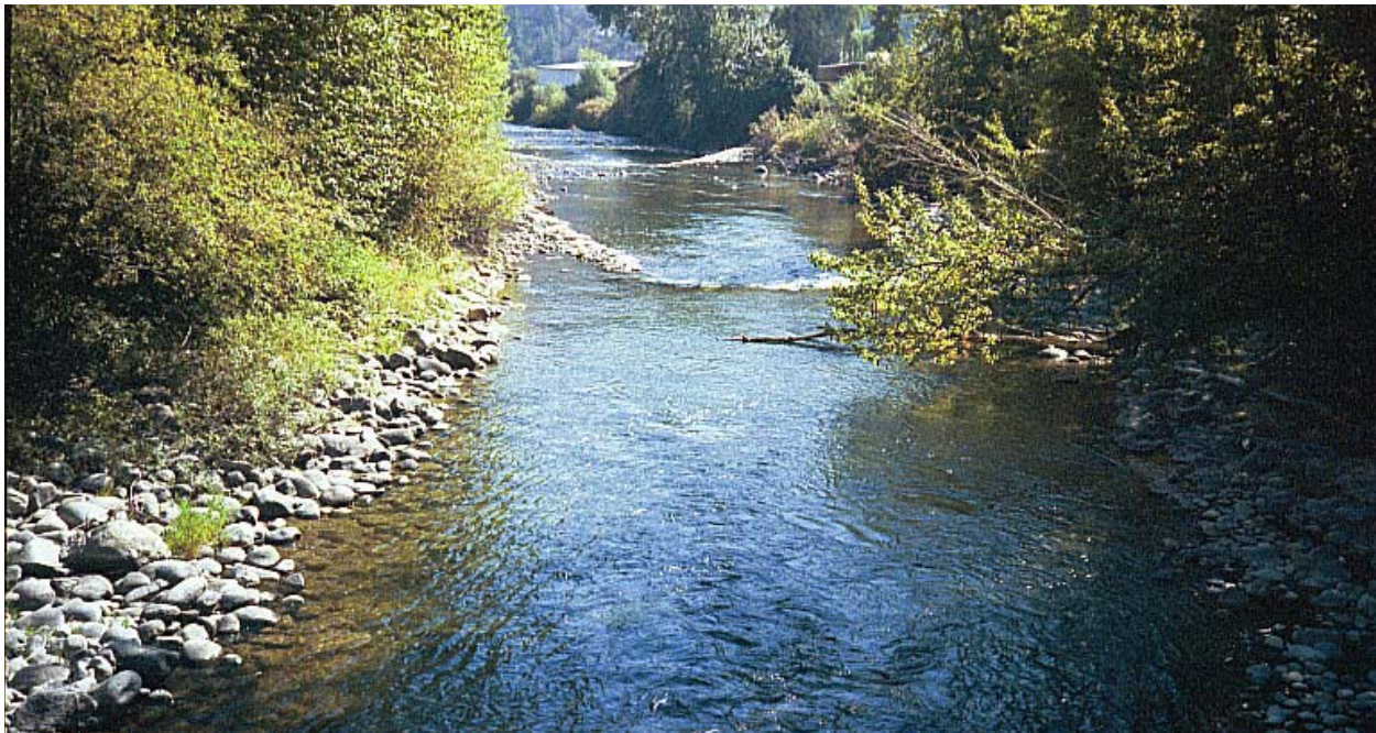
Figure 7-15. Looking downstream at two of rock cross vane structures installed in 2001 at the Fire Station Bridge site (RM 3.1).
